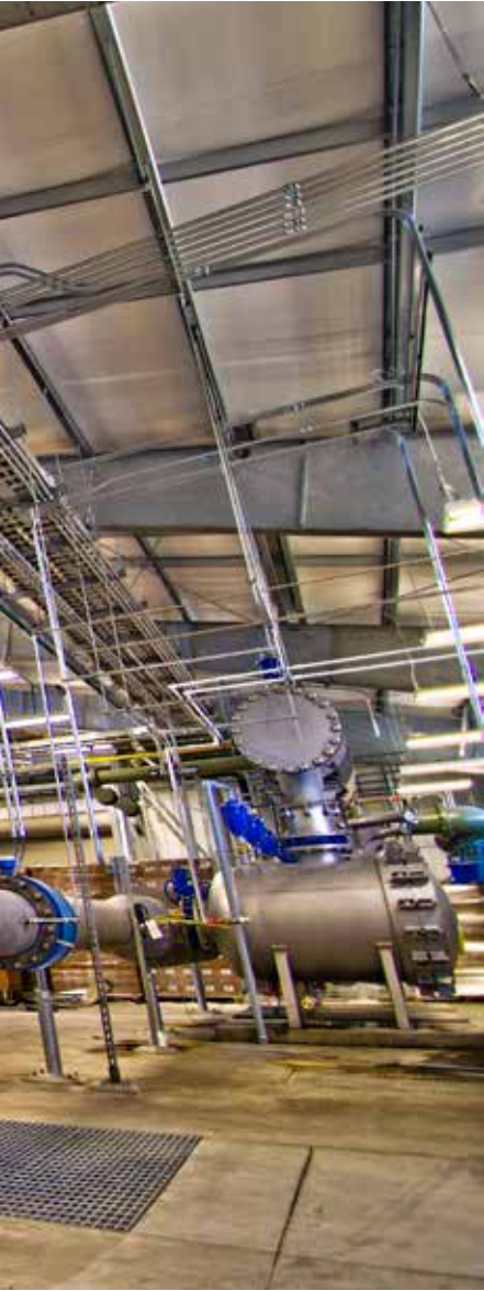
The award-winning reverse osmosis treatment plant uses deep injection wells to safely dispose of uranium-contaminated brine.
