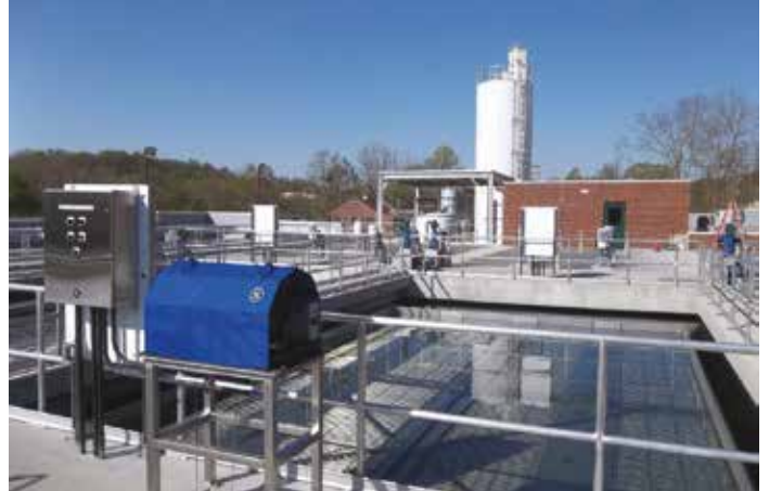
The use of BIM enabled the client to visualize every aspect of the water process.
