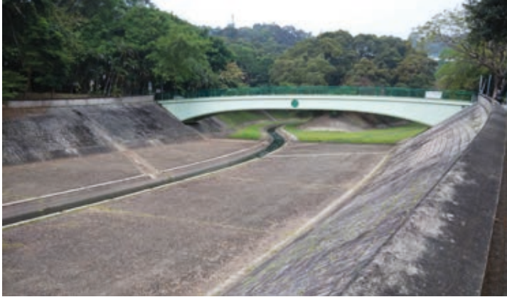
Figure 1 Site condition of Lower Lam Tsuen River before the ecological enhancement trial (Photo taken during 4th quarter of 2015)
